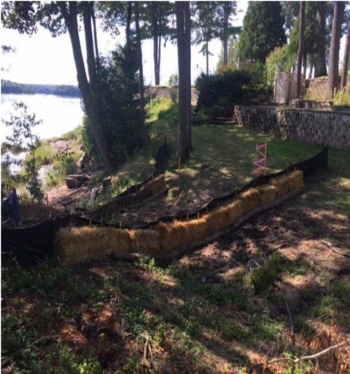
Fig 25: Second row of erosion controls installed downslope of man hole at Gundalow Landing. Viewing west. (8-29-19).
