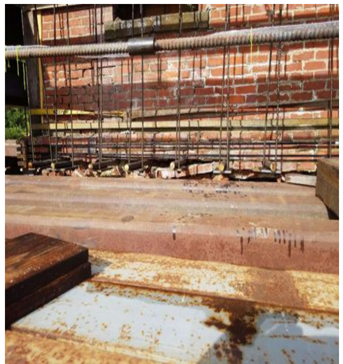
Fig 36: Cable house has been raised approximately 6in off of foundation. Viewing west. (8-29-19).
