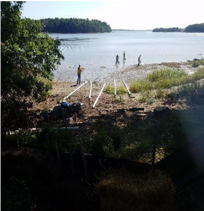
Fig 15: GZA installing PVC for treated water discharge into the Bay. Viewing south. (8-26-19).
