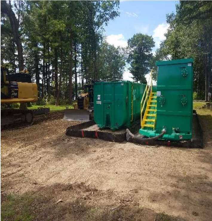
Fig 17: Water treatment tanks at Gundalow Landing. Viewing west. (8-27-19).
