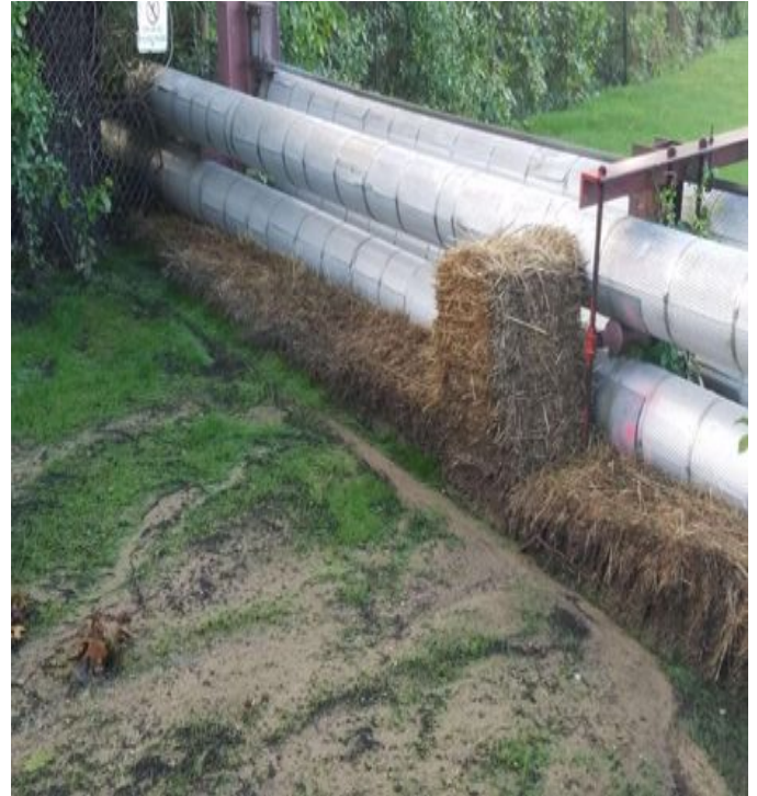
Fig 30: Erosion controls installed north of the steam pipe next to the field house at UNH. Viewing southwest. (8-29-19).
