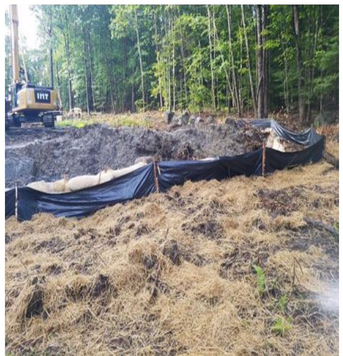
Fig 32: Erosion controls downslope of Str. 28 soil stockpile area. Viewing south. (8-29-19).
