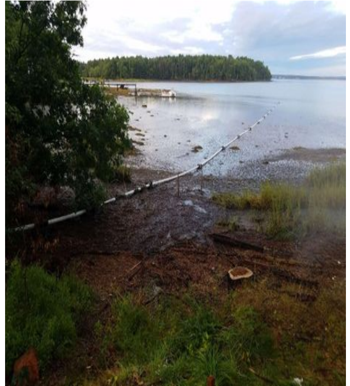
Fig 26: PVC discharge pipe installed in Little Bay for treated water. Viewing west. (8-29-19).
